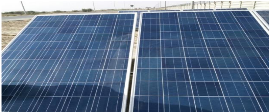
Figure 3. Dust removed PV modules
