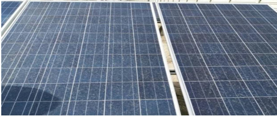
Figure 2. Dust accumulations on PV modules
